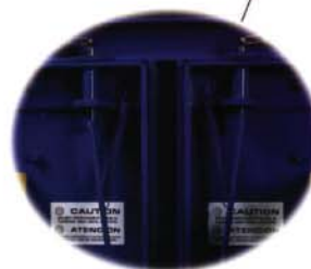
DOOR CLOSED WITH LIMIT SWITCH ACTIVATED.
